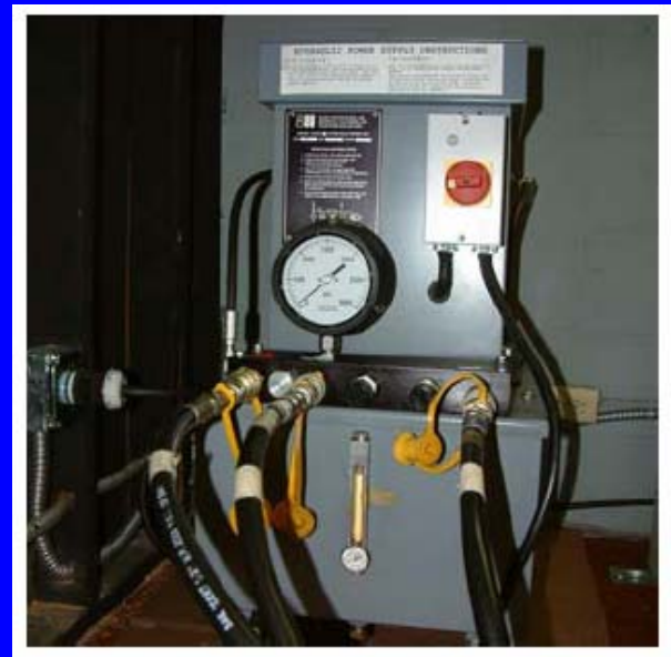
Hydraulic Power Supply
