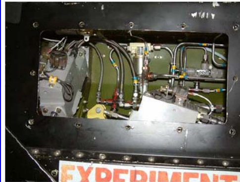
c) Hydraulic control loaders for EP station
